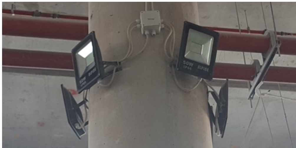
Figure 25: LED lighting fixtures on construction sites
