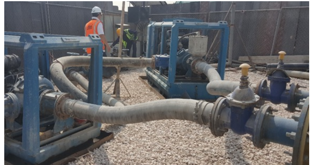
Figure 20: Energy-efficient dewatering arrangement on site
