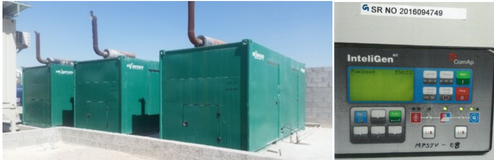
Figure 19: Generators Synchronizing System at Al Janoub Stadium
