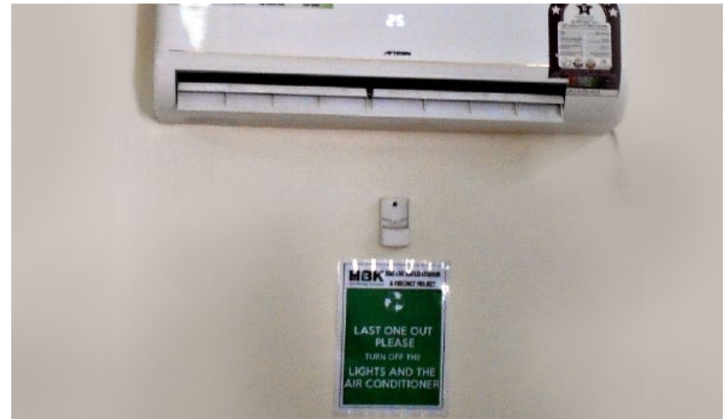
Figure 30: Staff reminder to turn off electrical systems
