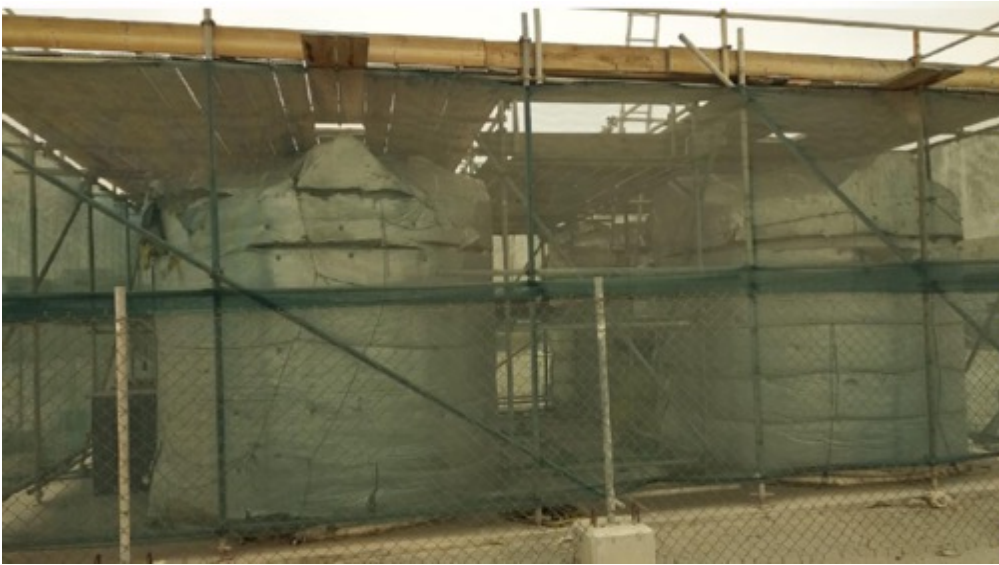
Figure 21: Shading and insulating of water tanks
