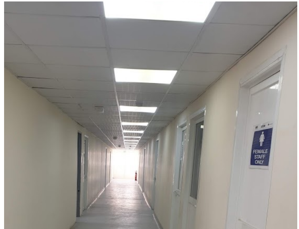
Figure 26: LED lighting fixtures in temporary buildings
