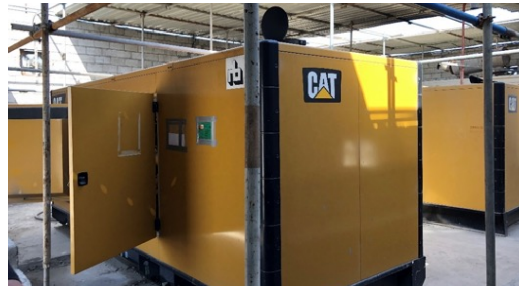
Figure 28: Example of diesel generator used on site
