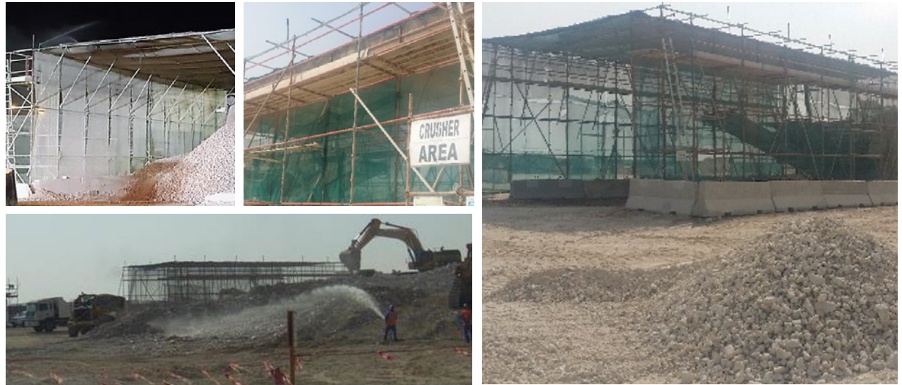
Figure 6: Suppression of dust from crusher
