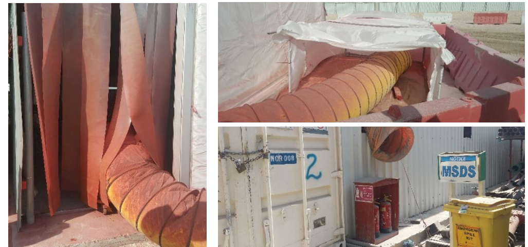
Figure 26: Indoor de-dusting systems
